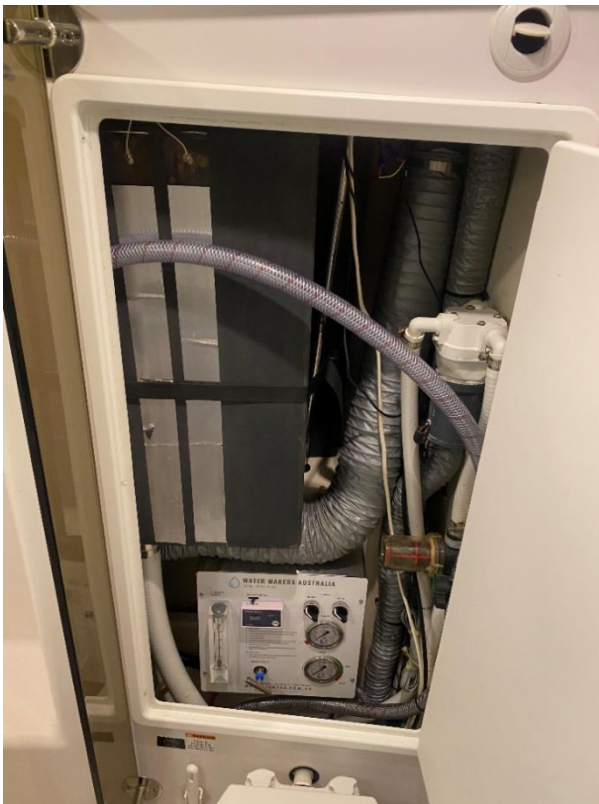
control panel in forward head
