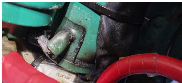
Burnt out starter motor
